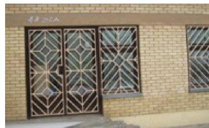
Picture 11. Thermal cold bridges (outdoor)
