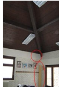
Picture 9. Thermal cold bridges (indoor)
