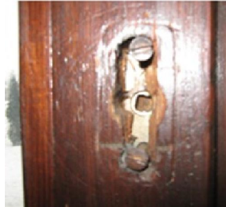
Picture 5. Inability of window opening
